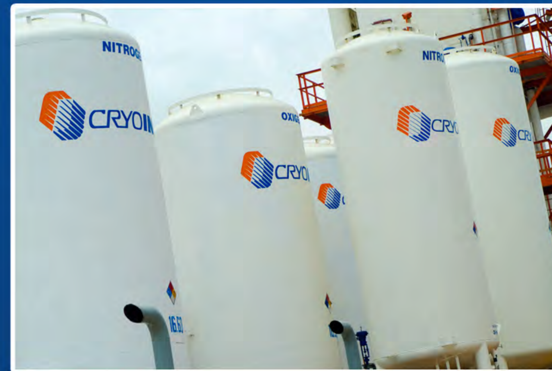
Liquid Backup Tanks
